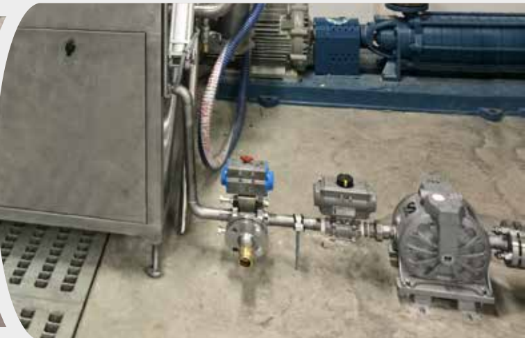
Chemical products dosing.
